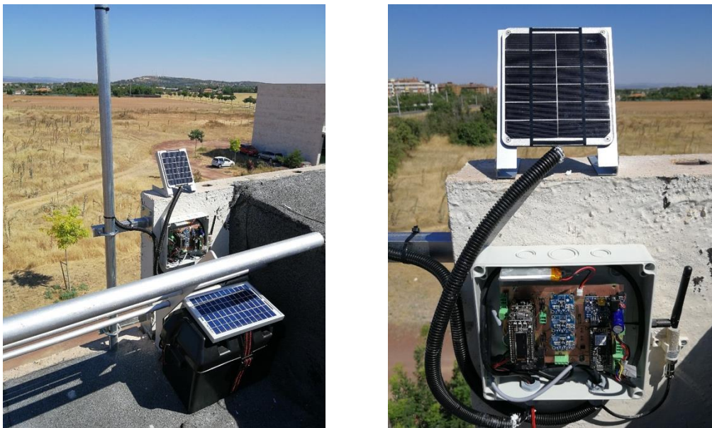
Figura 2 Deployment of our energy-harvested IoT prototype on top of a building of University of Castilla-La Mancha, Ciudad Real (Spain).
